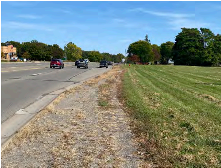
Aging and unkempt asphalt along edges of M-59
