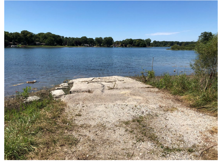
Photo 10: Remnants of concrete boat launch (to be removed) approximate location of proposed overlook/fishing pier.
