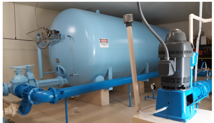
Pictured is Twin Lakes II Wellhouse on 5-16-2019.
